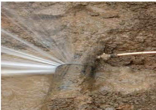
Fig 2: Leaking water pipe in Tanzania
