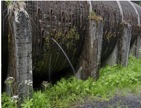
Fig 1:- Water leaks effects, photo credits John Fowler
