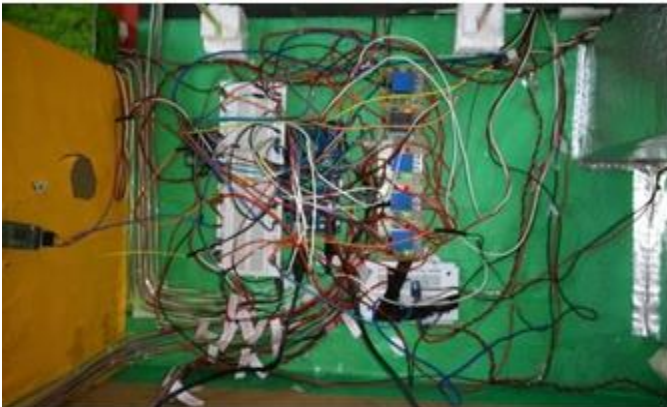
Fig 7:- Final Connection of the Project
