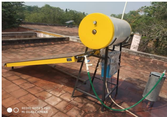
Fig.1:- Energy lab solar water heater connect to the energy storage setup
