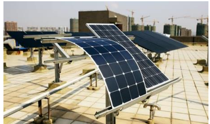
Fig3: show solar panel (thin film panels)
