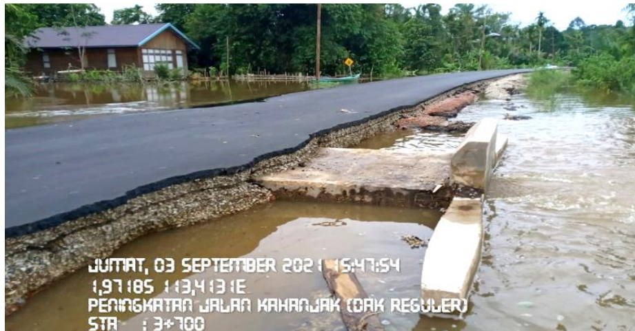
Fig. 3: The location of the Kahanjak Road Improvement Project (DAK-Regular) in TasikPayawan District in 2021 is flooded
