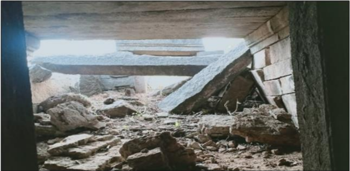
Fig 8 Poorly Damaged Arthamandapa of the 'Adi Narayanaperumal' Temple
