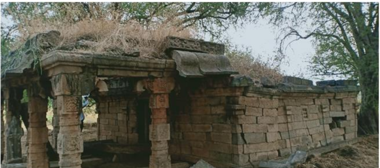
Fig 9 Damaged Side View of the 'Adi Narayanaperumal' Temple
