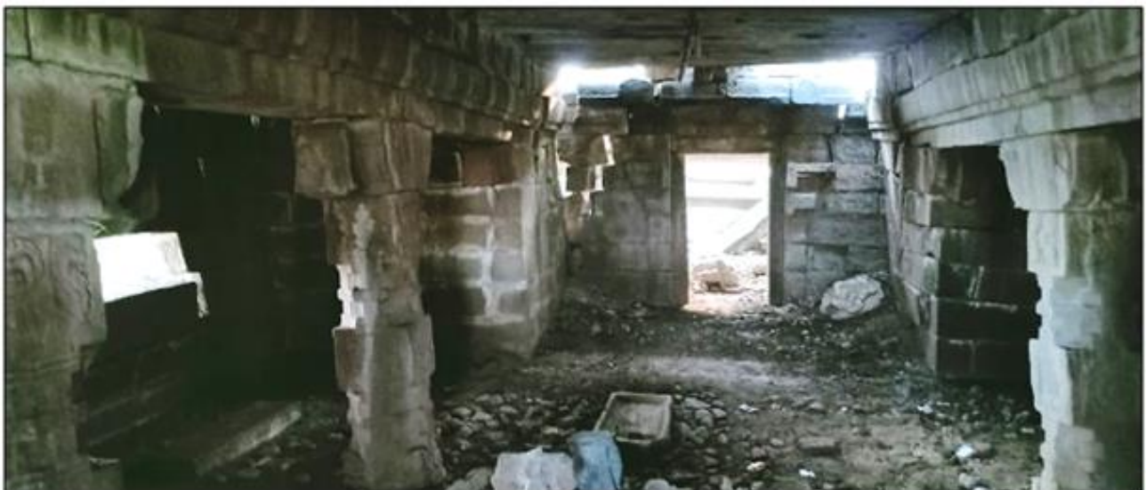
Fig 7 Badly Damaged Mahamandapa of the 'Adi Narayanaperumal' Temple
