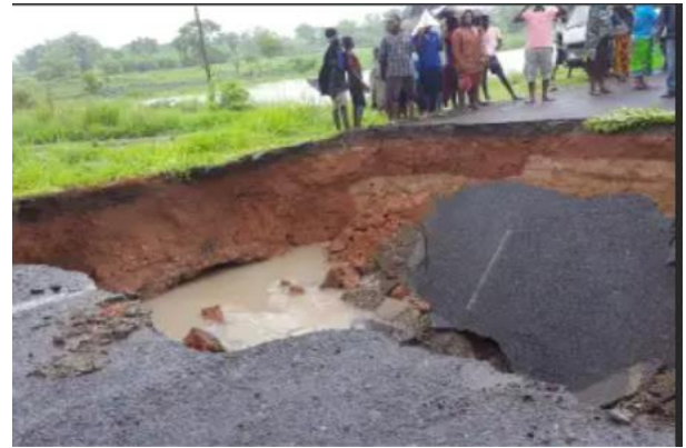
C. Damaged road
