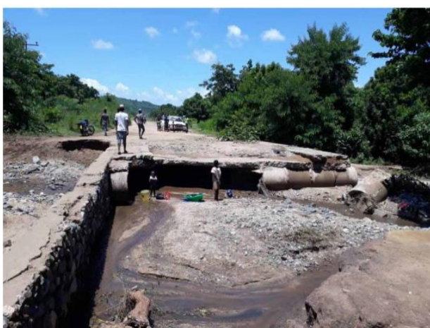
B. Bridge washed away
