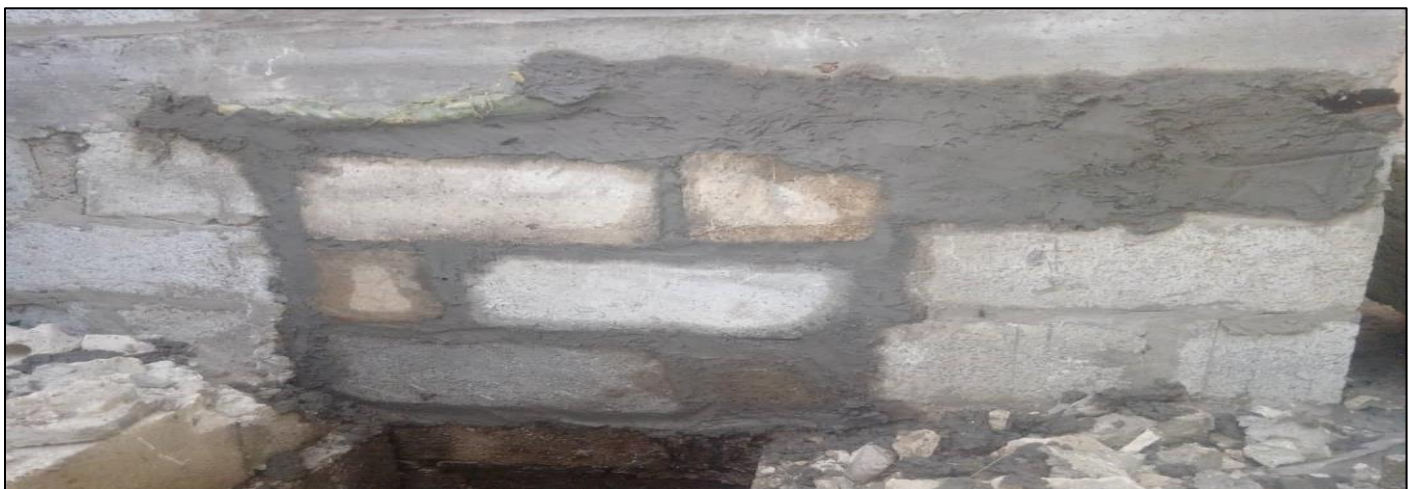
Fig 11: Mending of the Access Hole at the End of Collecting Solid Waste
