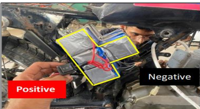
Fig 4 Battery Pack with a Preliminary Switch
