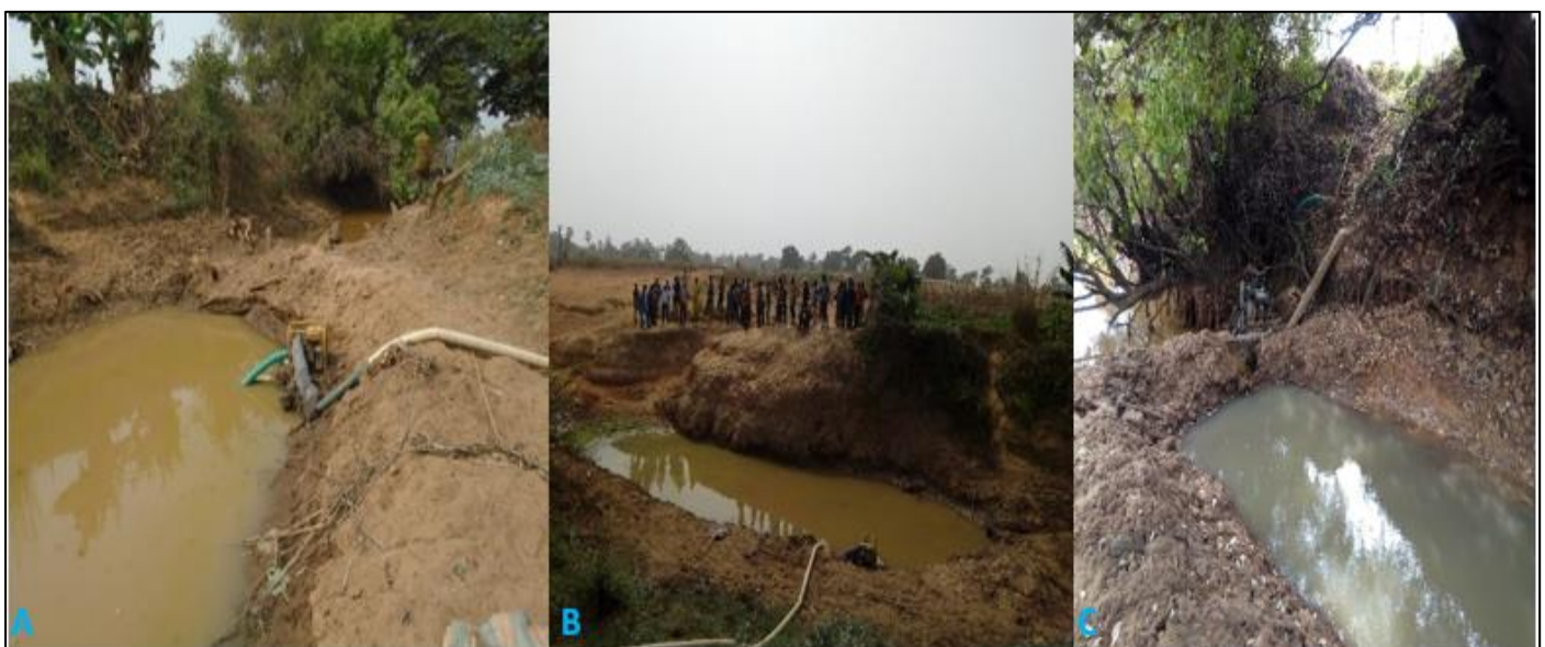
Photo 3: Development of Micro-Reservoirs in the Bed of the Comoé by Producers Photo: ZOUNDI M., April 2022
