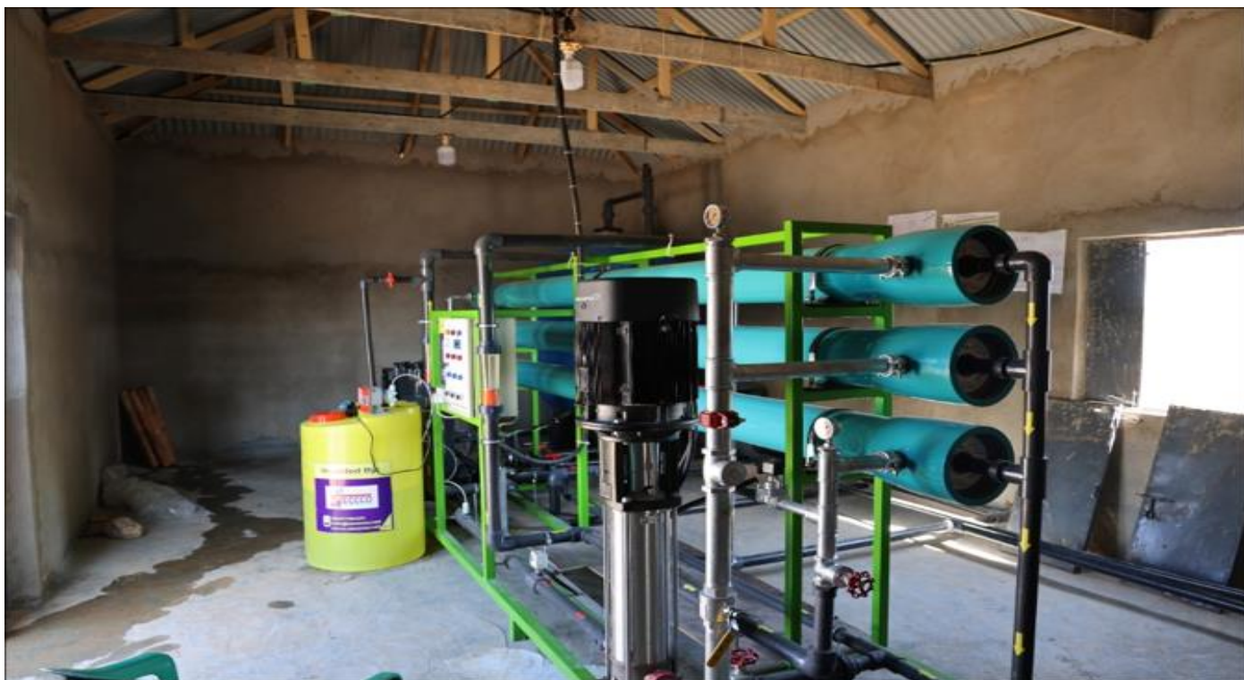
Fig 1 Installed Desalination Plant in El-dahir Village, Somalia
