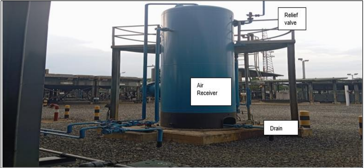
Fig 4: Showing Air Receiver, Relief Valve and the Piping and Instrumentation System
