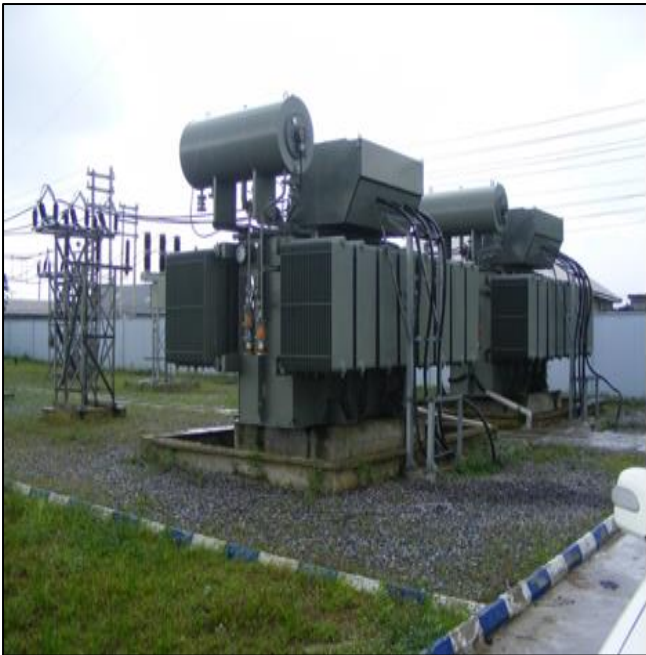
Plate 1.0: 33kV Iriebe Injection Substation (Source: Field)
