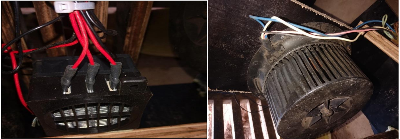
Fig 5: Fan and Heater
