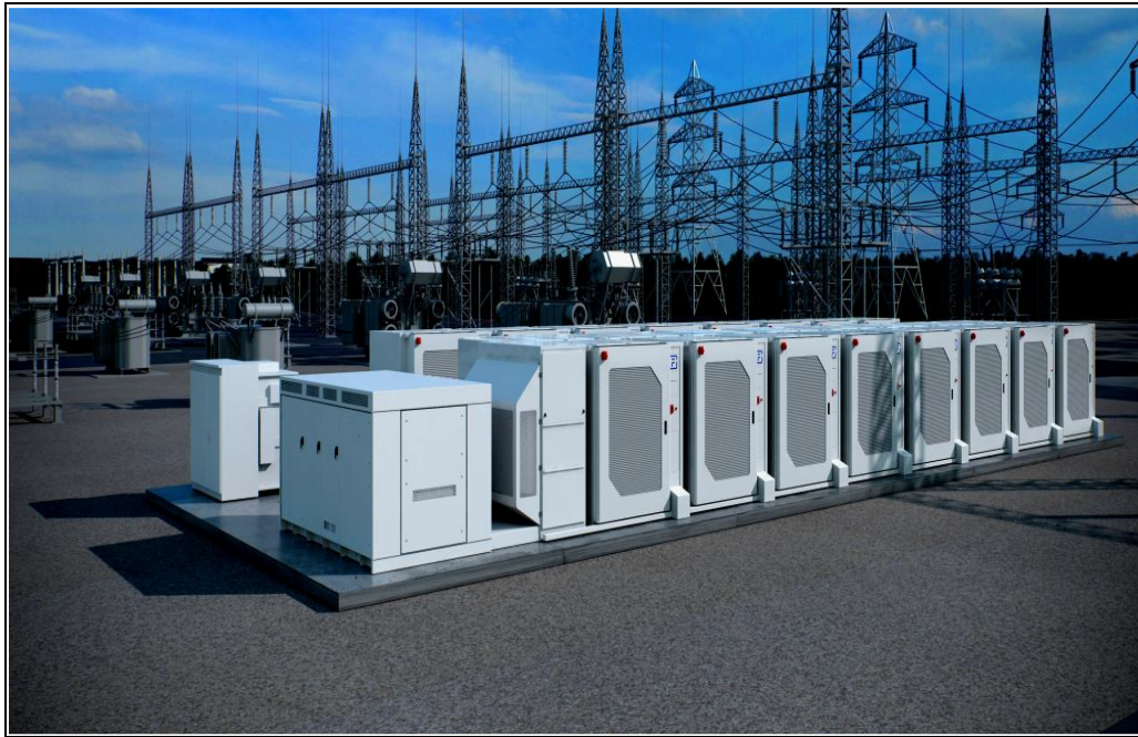
Fig 4 Battery Energy Storage Systems
