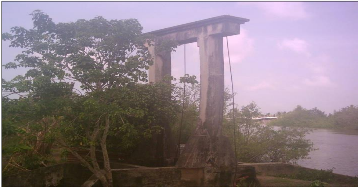
Fig 5 NATI Sluice on the South Bank of the Canje River
