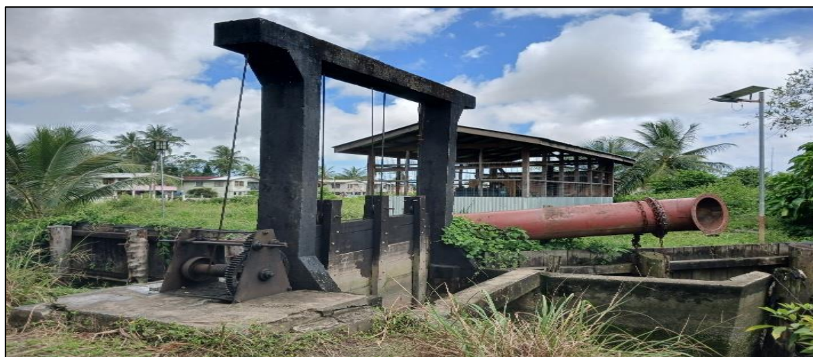
Fig 4 Tucber Sluice and Pump Station on the South Bank of the Canje River
