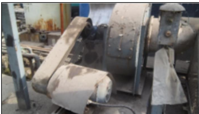
Photograph1 Degasser Blower Arrangement
