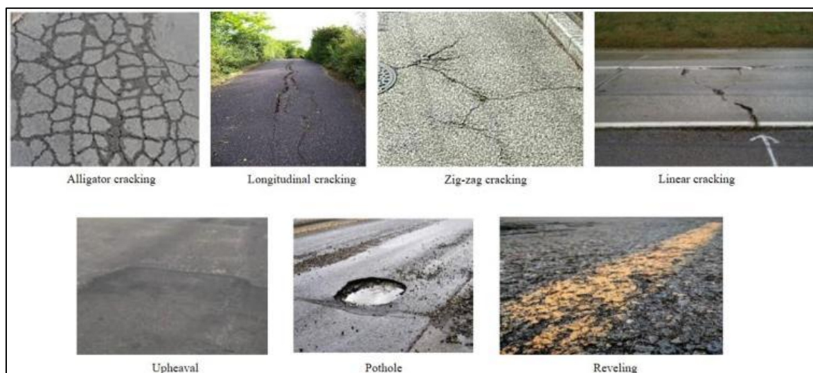
Fig 1 Road Damage Types with Samples for Detection
