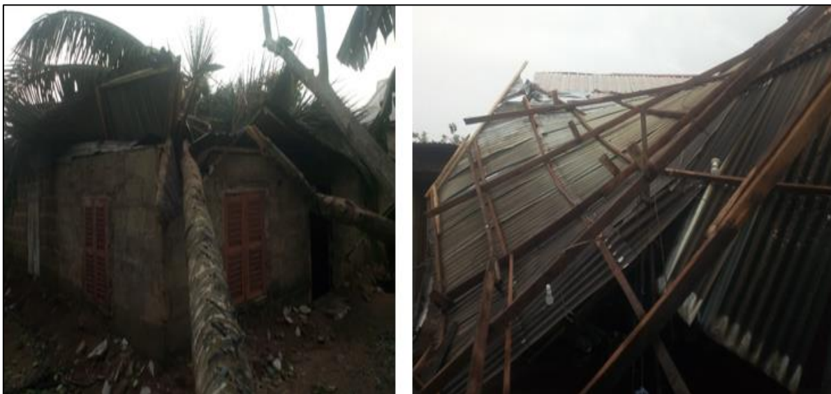
Fig 6 Structural Damage to Residential Buildings Following the Rainstorm
