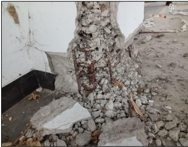
Fig 1 Severe Failure of The Structural Columns at The Tadulako University Hospital
