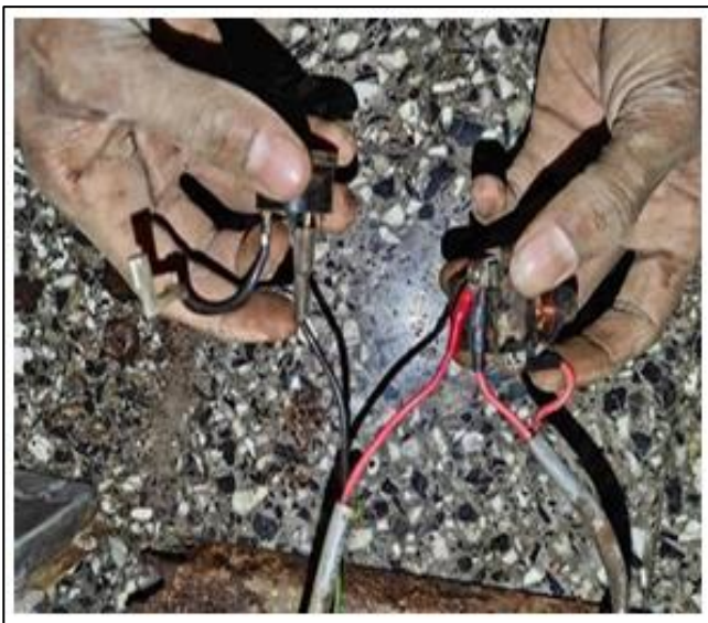
Fig 4 Faulty Relay Overload Removed from the System
