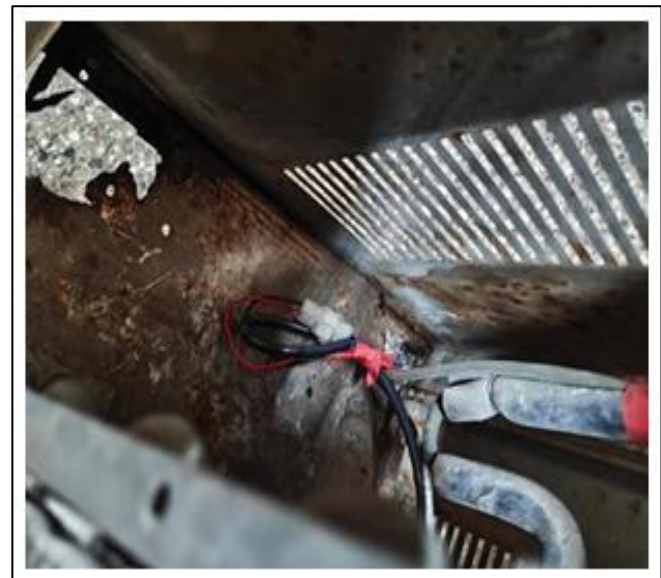
Fig 2 Rusted Base Sheet and Damaged Wiring before Repair
