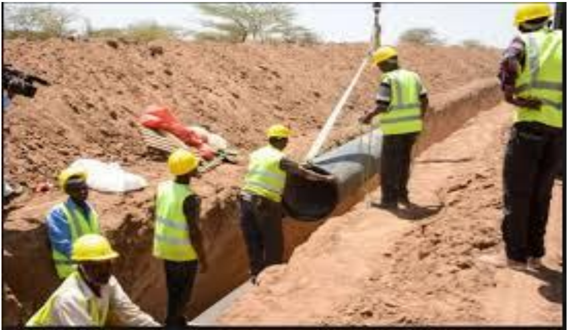
Hargeisa Water Supply Extension project Source: Field Observation
