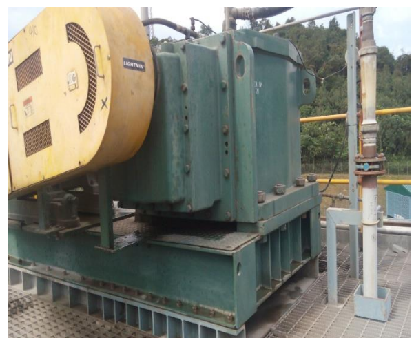
Fig 1:- Breather and Heat Exchange Connected to Agitator Gear box
