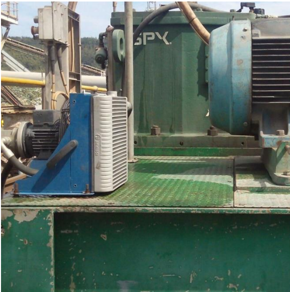
Fig 2:- Radiator Connected to Agitator Gear Box
