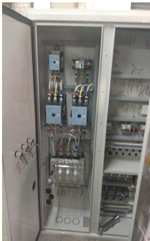
Fig 2:- Screw Chiller Control Panel
