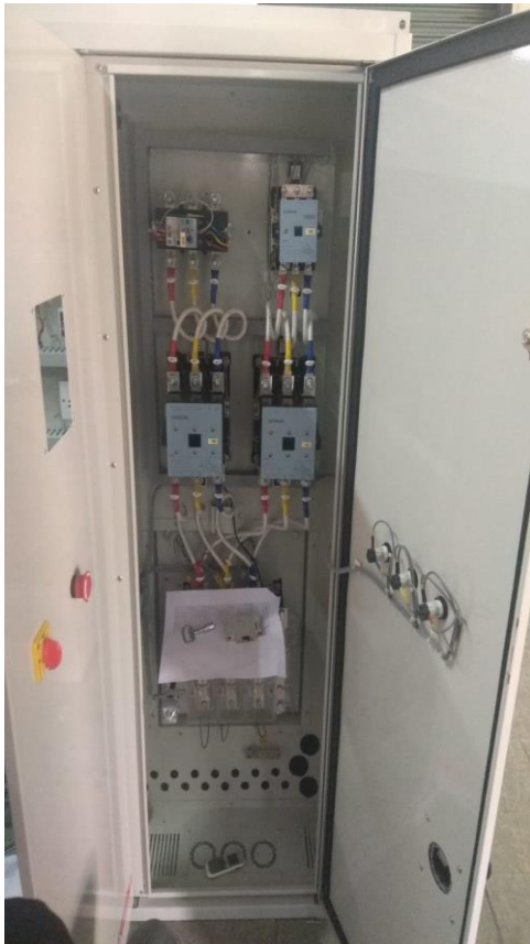
Fig 1:- Screw Chiller Control Panel
