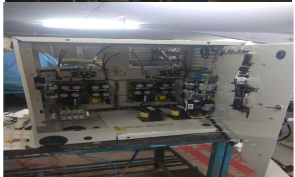
Fig 5:- Ducted Control Panel
